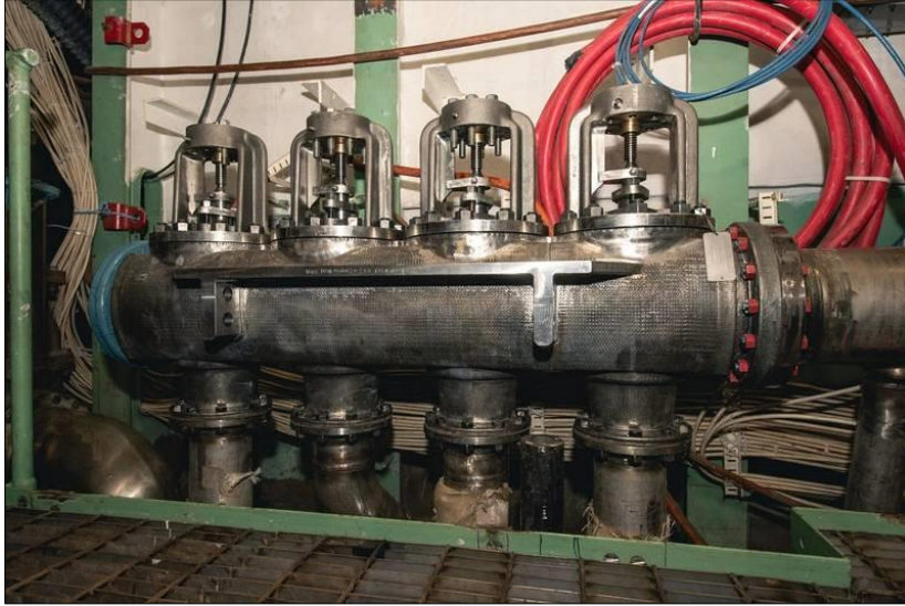
Figure 10. 3D Printed Valve Manifold Assembly for CVN-80 [62].
