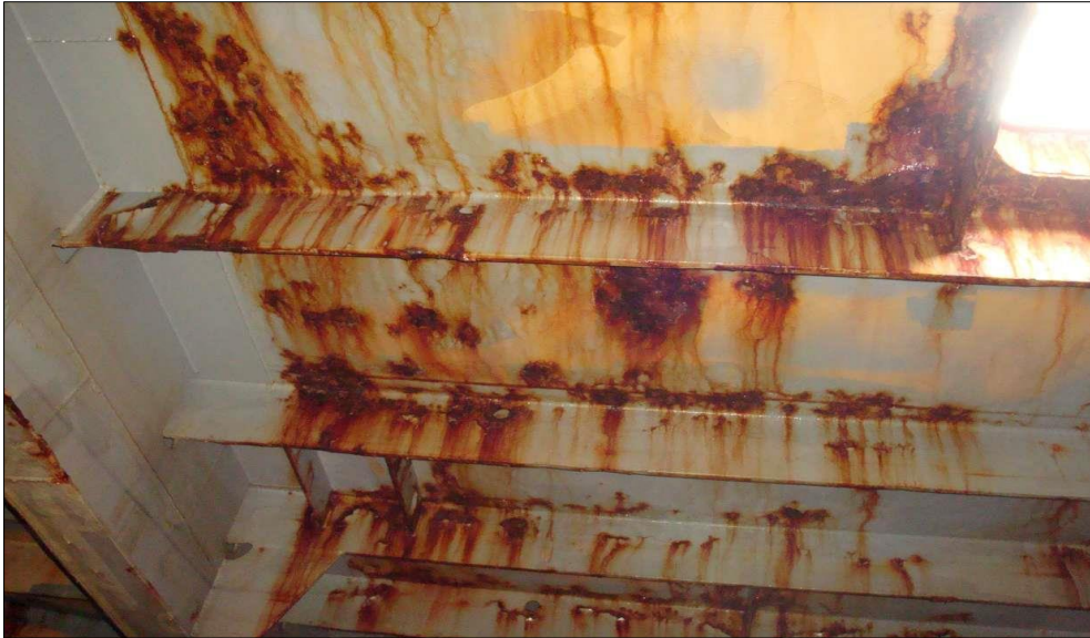
Figure 9. Severe internal corrosion observed in a ballast tank of a vessel. The image highlights extensive rust formation, coating failure, and pitting corrosion. Image source: Chemco International.
